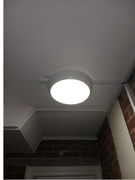
Lighting (Standard and Emergency Lights)
